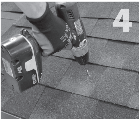
4 Using drill with 1/8" long bit, drill pilot hole into roof, taking care to drill square to the roof.
