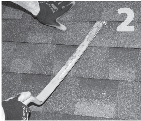
2 Lift composition roof shingle with roofing bar, just above placement of conduit mount.
