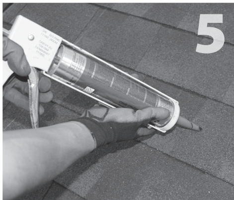
5 Clean off any sawdust, and fill hole with roof manufacturer's approved sealant.
