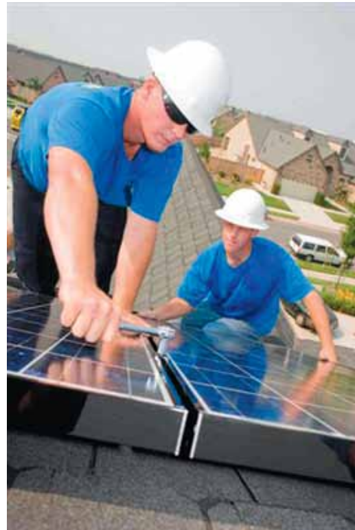
Check all bolts
