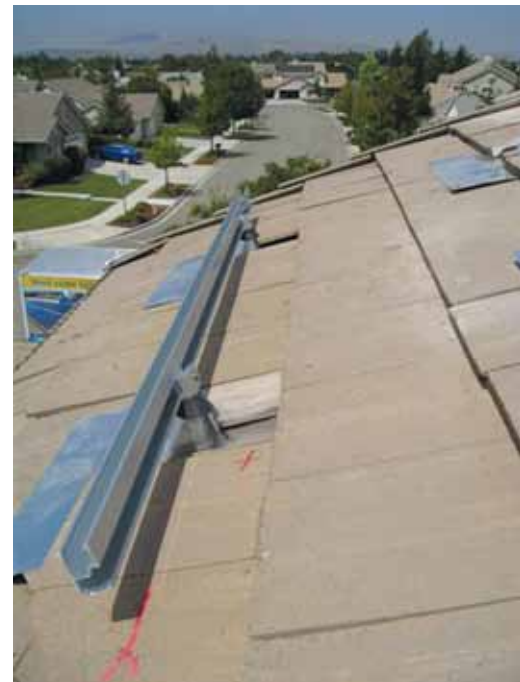
Fig 9.2 - Down-slope mounted rail
