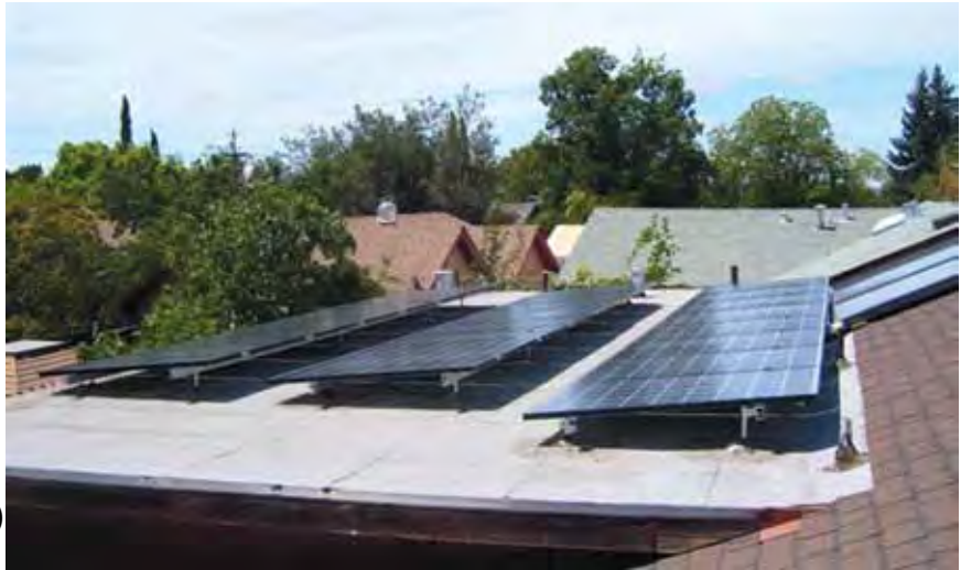
Fig 6.0 - PV modules installed at shallow angle
