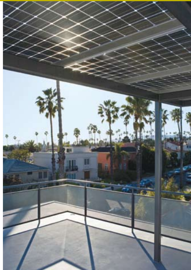
Rooftop Trellis: 1.95kW Golden Energy Inc. and Jesse Bornstein Architecture Santa Monica, CA
