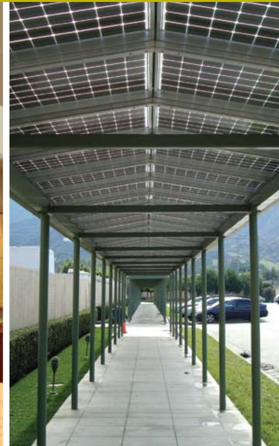
Breezeway: 44kW El Solutions Burbank, CA
